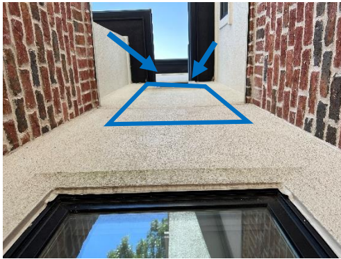
Photo 16.4 – kickout flashing missing
