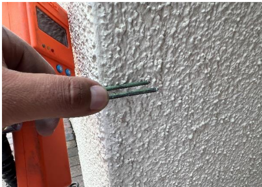
Photo 12.2 – prong extends past stucco and what would be the plywood
