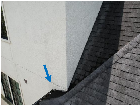
Photo 16.1 – kickout flashing missing
